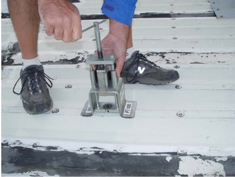
Figure 6: This picture shows Ron Olsen (Rain-Tite Roofing) measuring the pull-strength of typical fasteners used to attach the new roofing material. The pull strength of each fastener was typically 500 lbs. This is more than adequate to meet our extreme wind loads. Photo by Shawn Callahan (MMTO).
