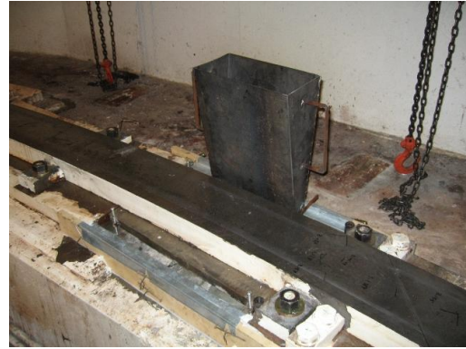
The track section alignment is verified, forms are readied for extruding cementitious grout under the track and sole plates.
